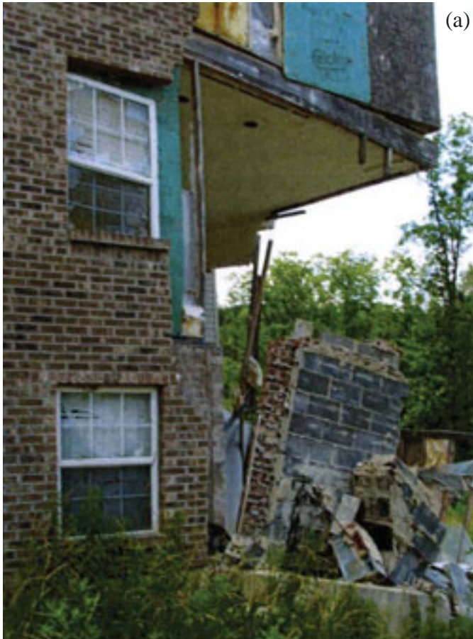
Figure 3.8 (a-e) Structural damage to homes can occur from hillside failure issues as illustrated by photographs of this home located on Rocky View Dr. in Campbell County. The building permit for the house was issued in 1996; the house was condemned in 2004.
