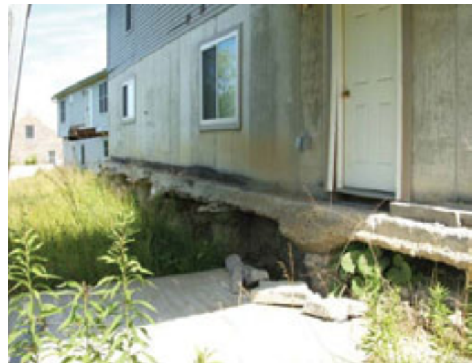
Figure 3.3 The dangers of poor hillside development; unstable slopes have compromised the foundations of several homes in Campbell County.
