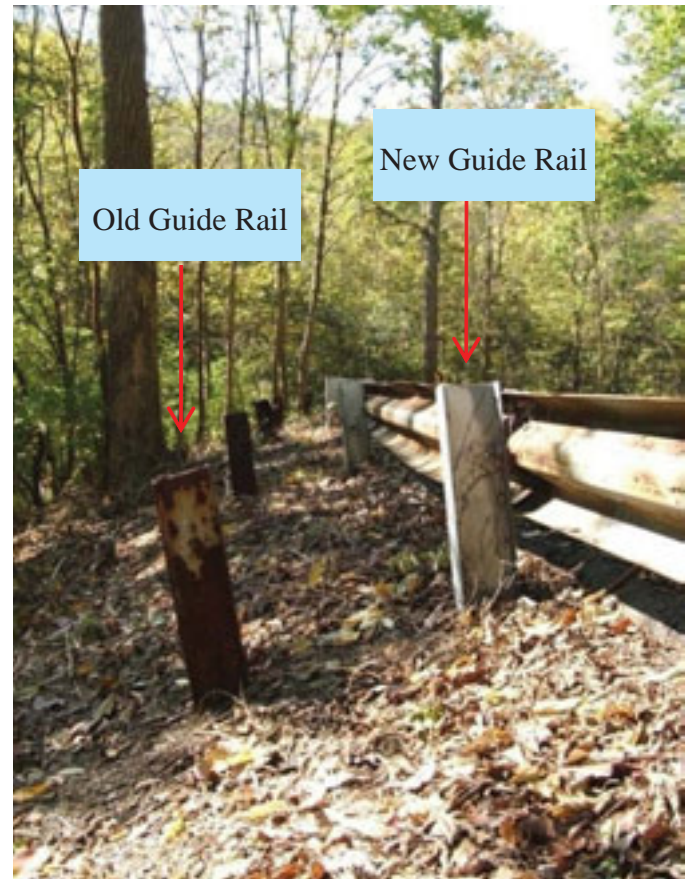
Figure 3.2 This guide rail along Sleepy Hollow Road shows signs of progressive downhill sliding.
