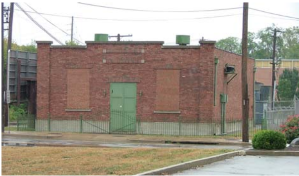
Figure 4.5.7: Duke Energy Substation
