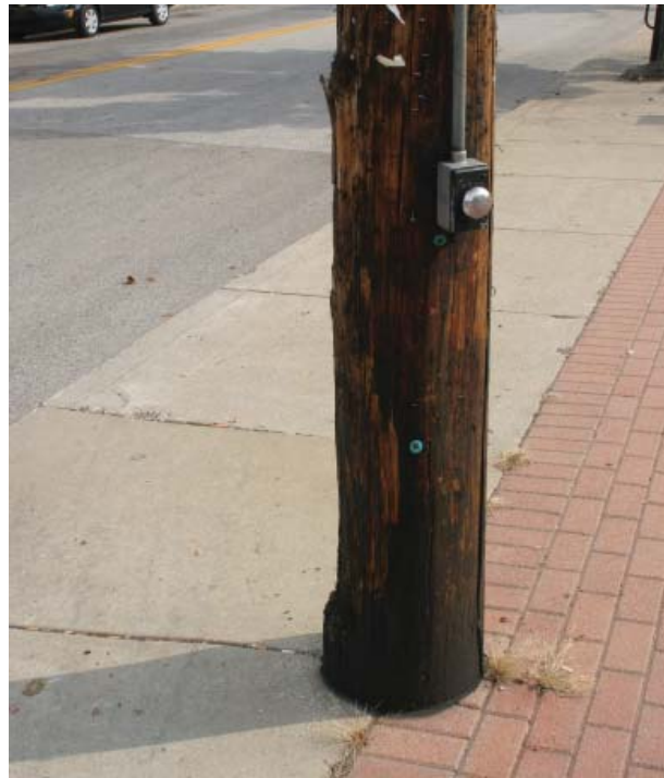
Figure 4.6.5: Utility Damage in Ritte's Corner
