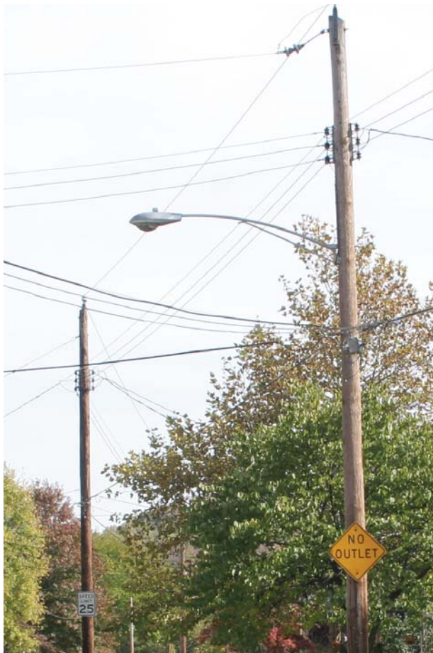
Figure 4.7.1: Standard Utility Lights
