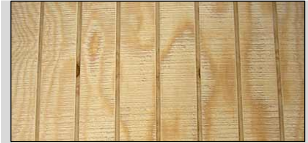
Above: Weak and fragile building materials do not adequately withstand the elements and quickly deteriorate leaving an unsightly appearance
